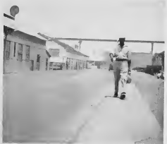
This man is walking where tube bundles will be repaired and tested when the addition to the old shop building is finished. This section (see 9 on drawing on page 4) will be 3,500 sq. ft. of storage space. Pipe and welding shops at left were dismantled.
